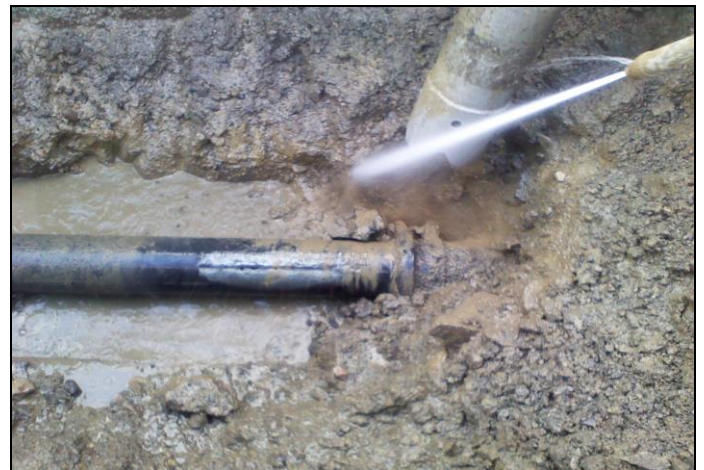
Water main break on South Main Street.
