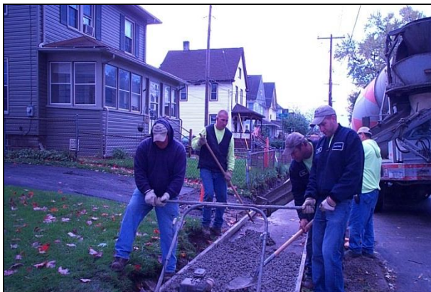
2011 sidewalk improvements on Montclair Ave. is an example of work done by City staff.
